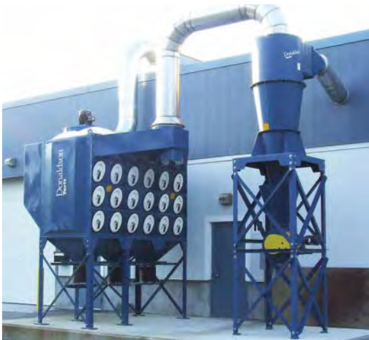
DFO & Cyclone on Thermal Spray 4,800 cfm (8,154 m 3 /h)
