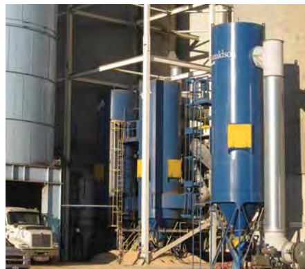
RF - Grain Terminal 34,000 cfm (57,754 m 3 /h)
