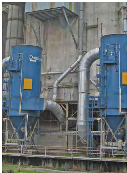
RF - Grain Terminal 61,000 cfm (103,618 m 3 /h)
