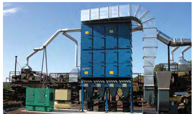
DLMC on Rock Crushing 41,000 cfm (69,645 m 3 /h)
