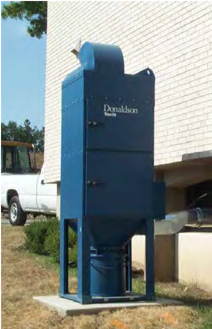
UMA - School Wood Shop 2,000 cfm (3,397 m 3 /h)
