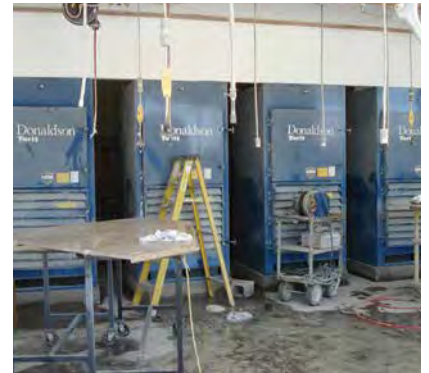
DWS on Granite Finishing 22,000 cfm (37,370 m 3 /h)
