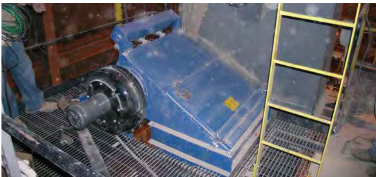
CPV - Bucket Elevator 1,200 cfm (2,038 m 3 /h)
