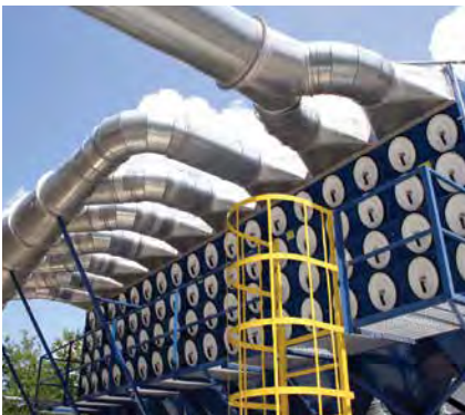
DFO on Sawdust 57,500 cfm (97,692 m 3 /h)
